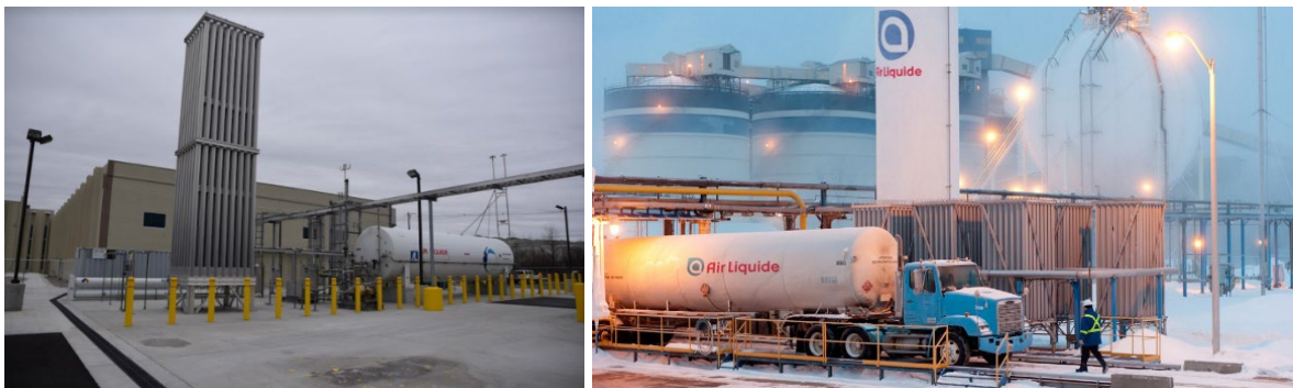
Figure 22. Air Liquide LH 2 filling stations (left: Little Town, USA; right: Becancour, Canada).
