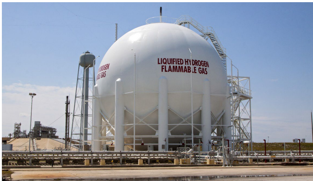
Figure 26. LH 2 storage vessel with 3800 m 3 capacity at KSC in Florida (Source NASA).
