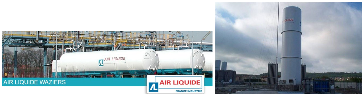
Figure 24. Horizontal and vertical liquid hydrogen storages. (Source Air Liquide).
