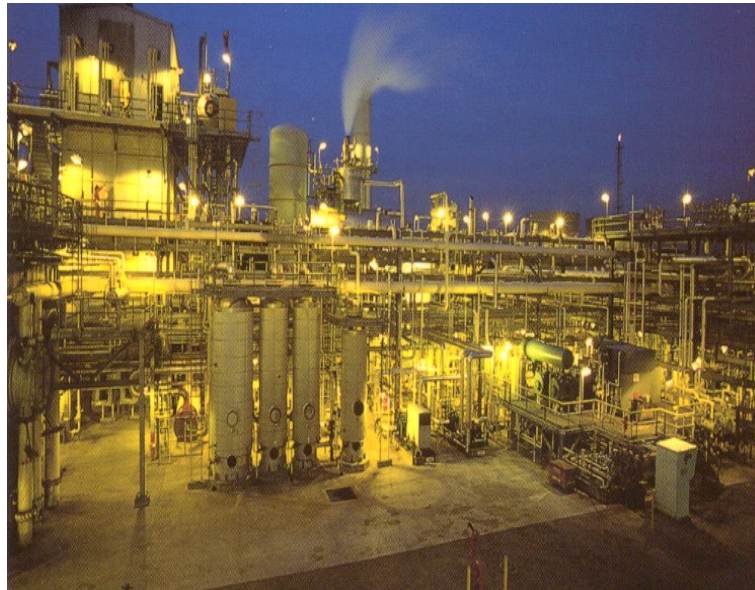
Figure 30. Air Liquide SMR plant.
