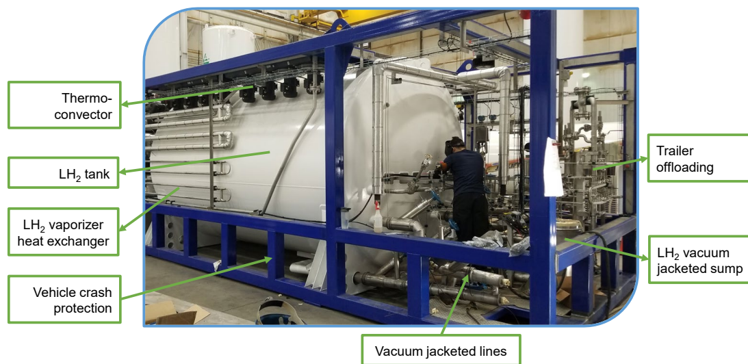
Figure 13. LHRS skid overview – “Cryogenic” side.
