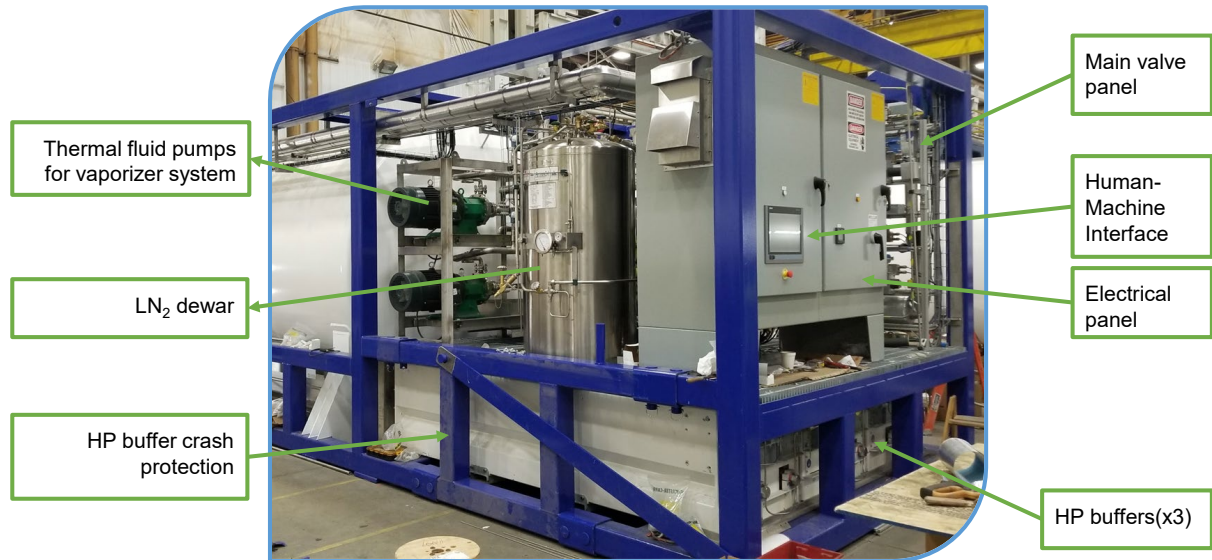
Figure 14. LHRS skid overview – “Warm” side.
