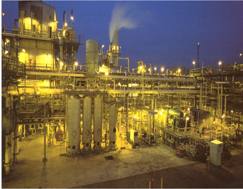
Figure 30. Air Liquide SMR plant.
