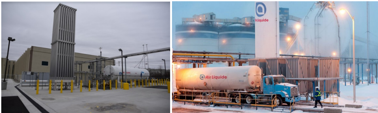
Figure 16. Air Liquide LH 2 filling stations (left: Little Town, USA; right: Becancour, Canada).
