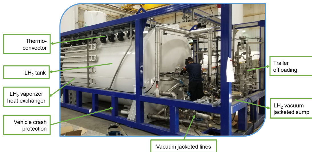
Figure 13. LHRS skid overview – “Cryogenic” side.
