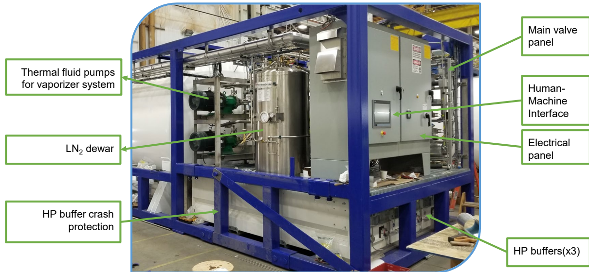
Figure 3. LHRs skid overview – “Warm” side.
